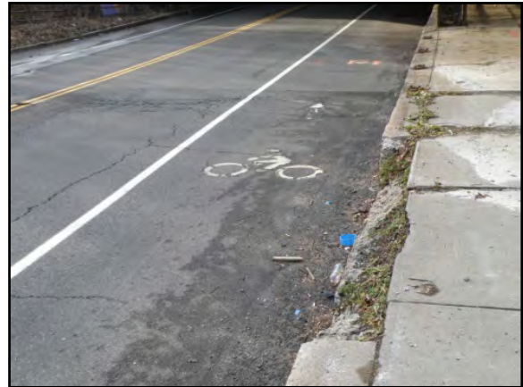
Fading Bike Lane Markings on Capitol Avenue
